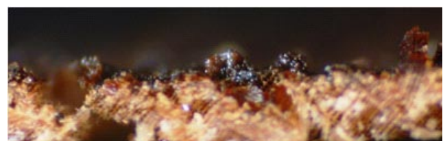
Figure 7 Transverse section taken from surface of western red cedar cladding with severe extractive staining, showing dark-coloured extractives confined to the surface zone
