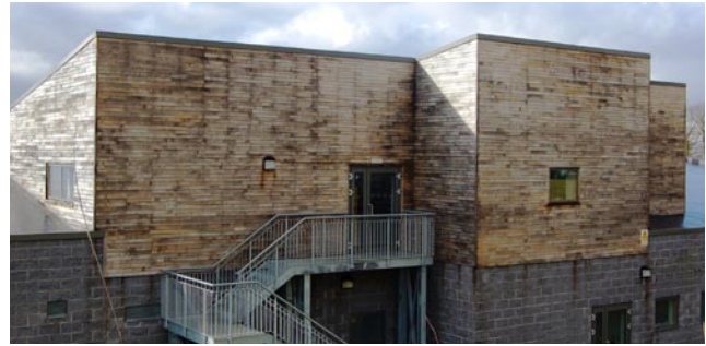
Figure 5 Dark vertical lines on open-jointed sweet chestnut cladding
