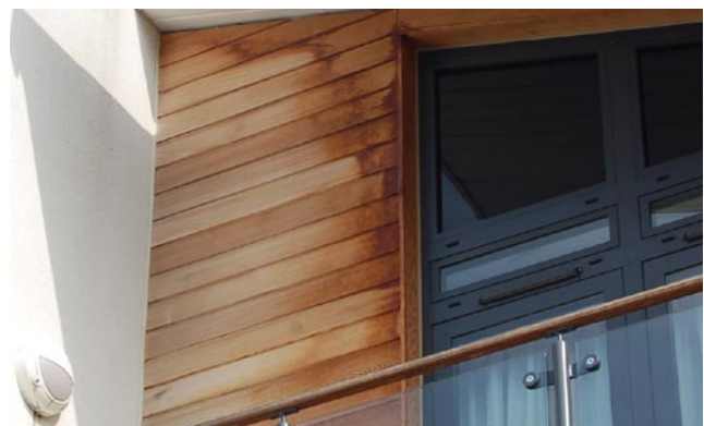
Figure 6 Extractive staining on western red cedar beneath break in eaves canopy
